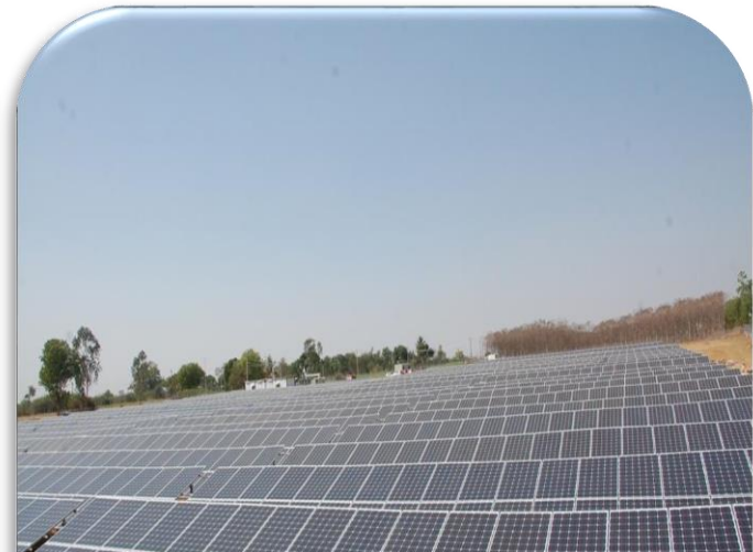
SOLAR POWER PLANT, MUKTYALA – 1.15 MW
